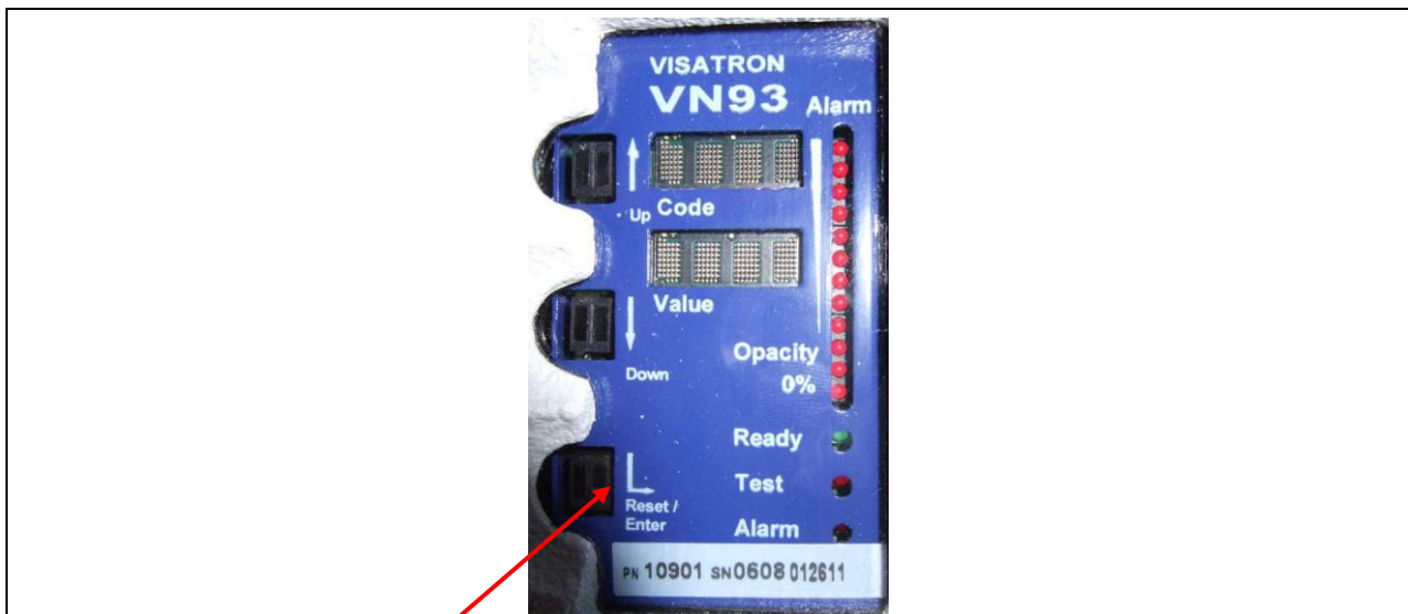
Figure 41: Oil-Mist-Alarm reset light button
